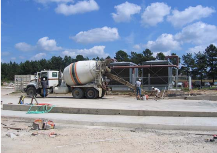
Pouring Sidewalks on north side of McCurtain Memorial Hospital on September 23rd.
