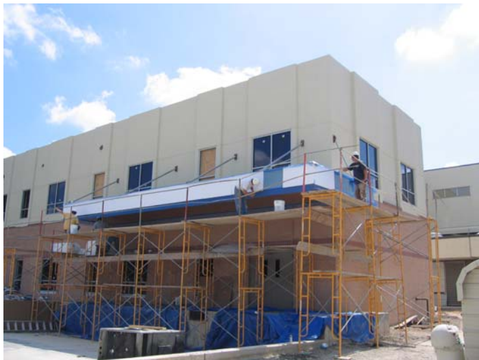
Construction Workers continuing to install efis on the North Tower on September 23rd.
