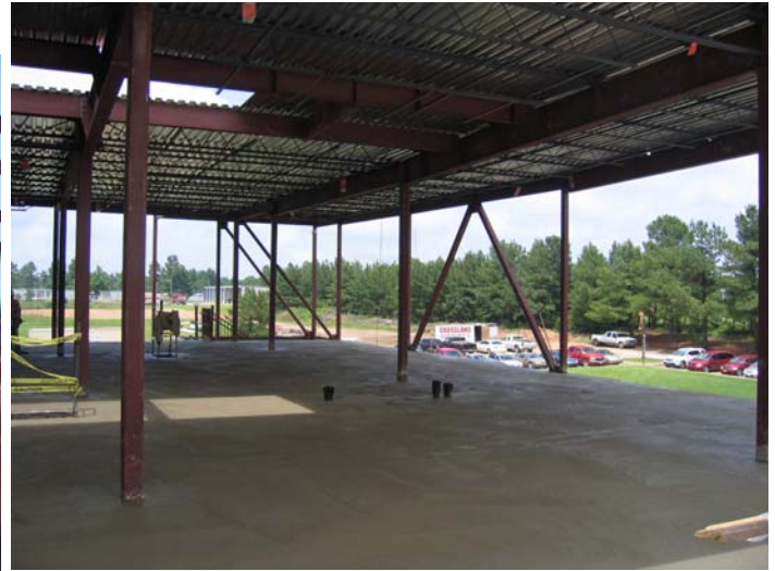
Concrete was finished on the 2nd Floor of the North Tower Construction on June 10th
